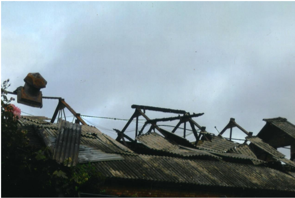
The remains of the auditorium roof after the fire, this was a view that would be seen for years after the fire.
